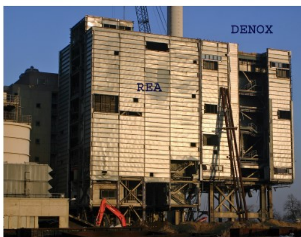
Fig.2 Power Station View Two
