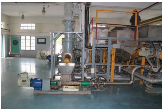
Fig. 3 Typical View of PCP pumps with safety cutoff
