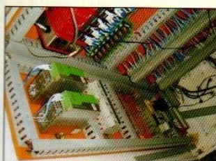
Automation and Control
