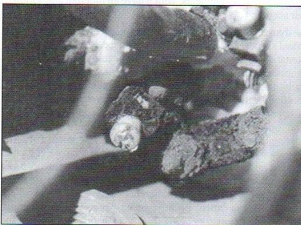
Figure 2 - Crystals of tetrammine copper (II) nitrate formed by the interaction of AN with copper in an electrical box in an explosives plant.
