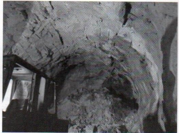
Figure 5 - Tunnel Profile with Minimum Overbreak after Application of New Blasting Techniques at LNPHEPP
