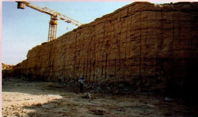
Pre-split blasting by NIRM at a Nuclear Power Project (15m high wall)
