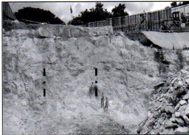
Figure 9 - Face made in the Station area for Launch of TBMs for Twin Tunnels
