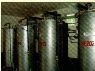
Continuous MMAN Plant
