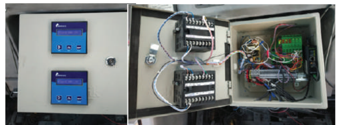
Figure 11-Photograph of the control unit
