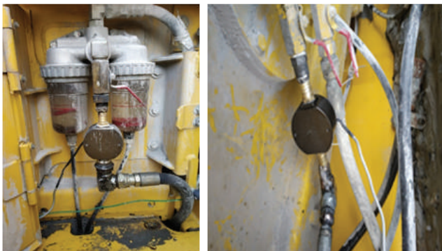
Figure 9 - Sensors fitted in diesel supply line (intake and return)
